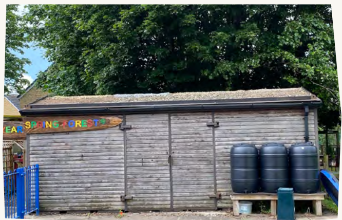
Green roof suitable for ground-nesting birds and with water filtration system
